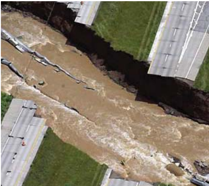
Figure 1 Aerial view of the I88 Carrs Creek culvert failure.
