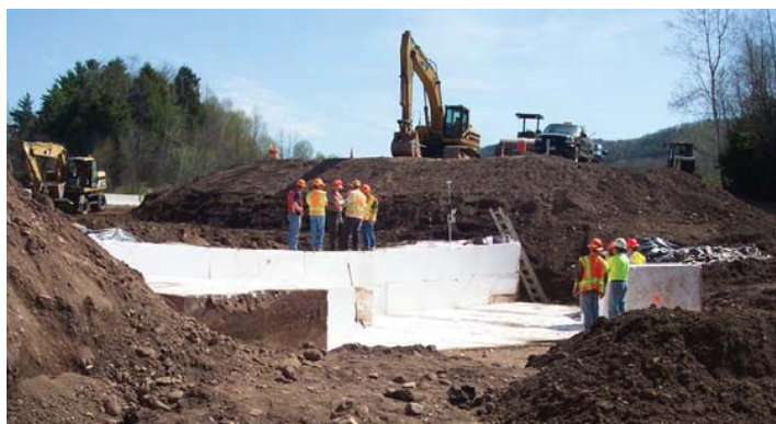
Figure 2 Excessive settlement and removal of the geofoam fill.
