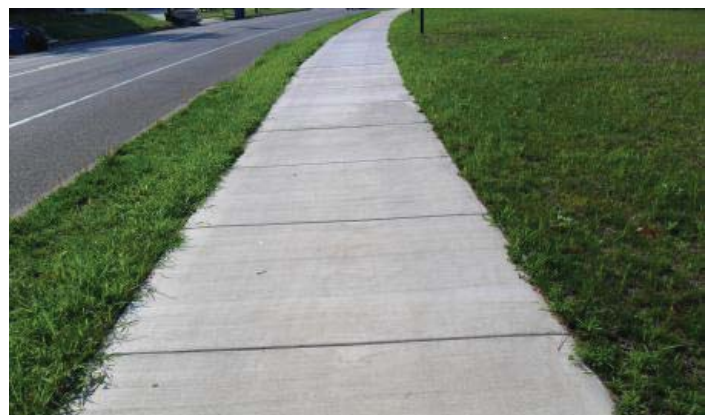
Figure: Carpenter Street placement on June 30, 2011 and condition on Aug 9, 2012
