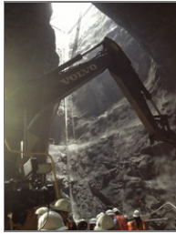
This is a look up from the 86th Street Station construction site.
